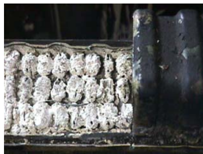
Solder bloom caused by degradation of the rust and corrosion inhibitors and oxidization of lead in the solder
